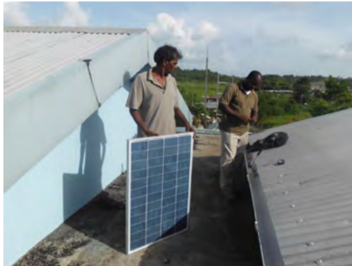
Solar panel installation for disaster shelter at the Rochard Douglas Presbyterian School, Barrackpore
